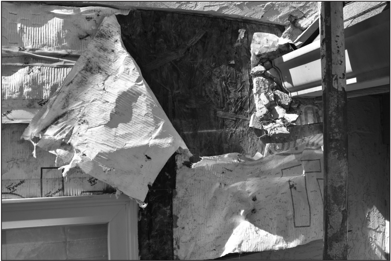
Figure 1 - Damaged sheathing resulting from improper building product installation
